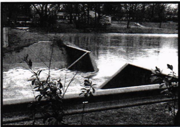
Full Flowing V-Notch Weir Stormwater Detention System (MTG)
